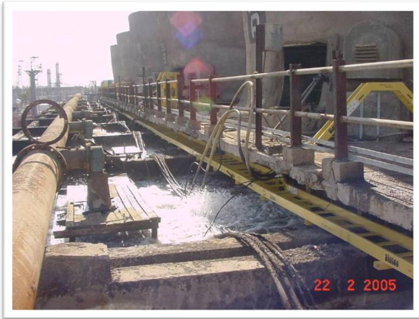
Cooling Tower @ IOCL Baroda
